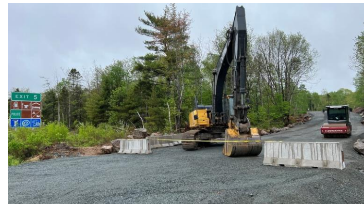
New emergency exit following Tantallon wildfire
