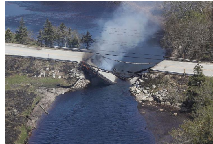
Collapsed bridge from Shelburne wildfire
